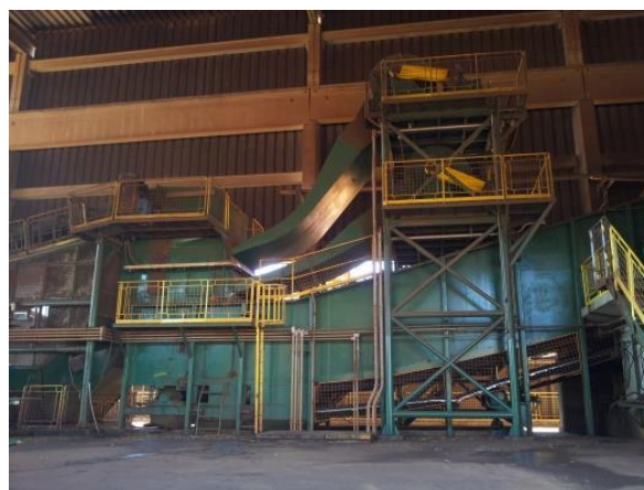
Figure 2. Dry cleaning system in Alta Mogiana sugarcane plant.
