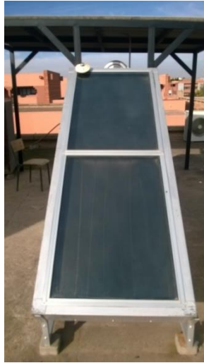
Fig. 6. Front view of the utilized flat plat solar air heater.
